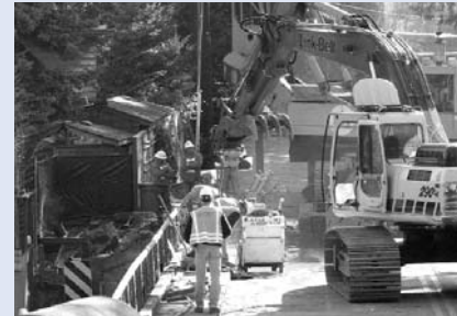
Construction has begun on the new Oswego Canal Bridge, which will remain closed through December.
