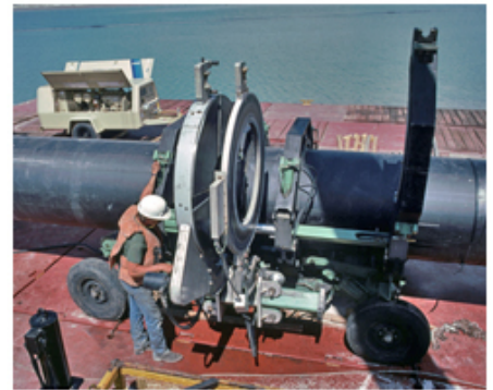
Pipe fusing will begin from the dock near Oswego Dam in the fall.
