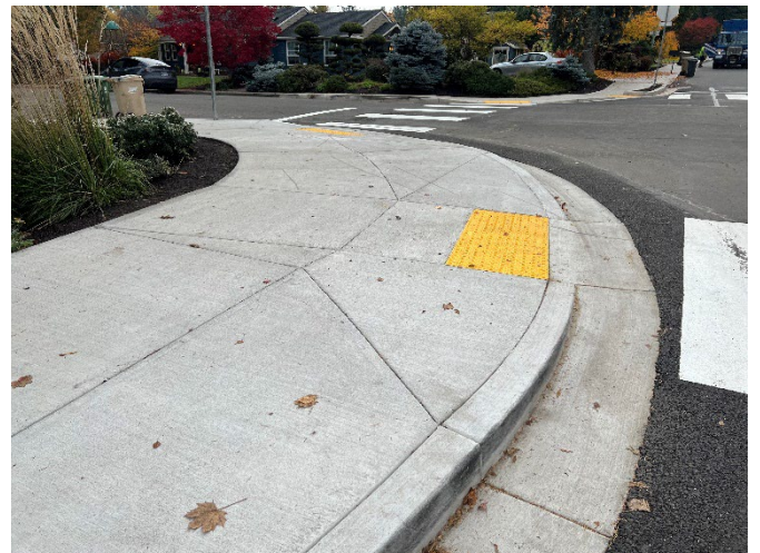
Picture 5: A new ADA-compliant curb ramp and crosswalk have been installed at the intersection of Hallinan Street and Hemlock Street, improving accessibility and safety for pedestrians.
