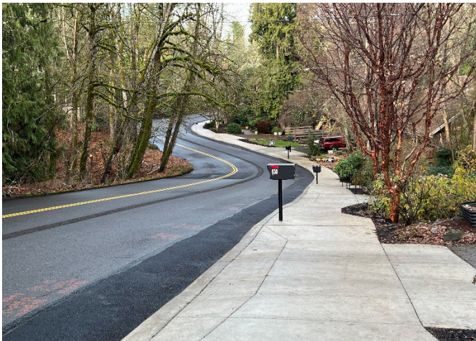
Picture 4: A new ADA-compliant sidewalk was completed on Boca Ratan Drive in 2023, enhancing accessibility for pedestrians.
