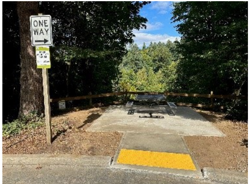
Picture 9: A new curb ramp has been installed at Tryon State Park, providing accessible access to the picnic table.
