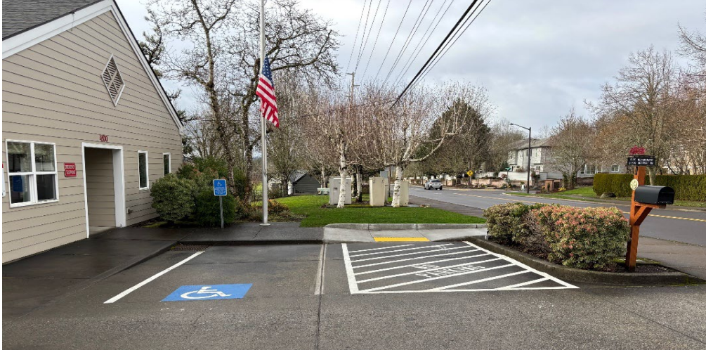
Picture 4: Freshly repainted parking space, access aisle, and ADA emblem, along with a newly installed curb ramp at Westlake Fire Station.
