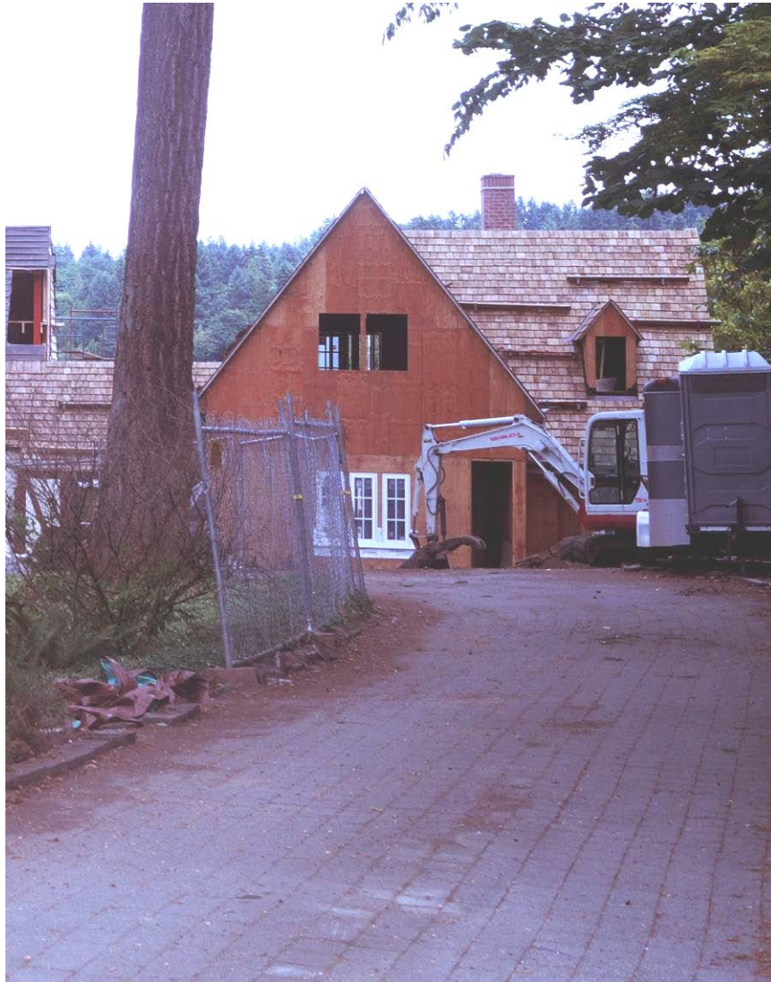
Figure 7: looking east at the west façade. Note this is new construction (new wing), March 2014
