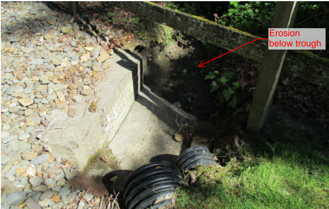
Area 3.6 - Outfalls into concrete trough with significant erosion downstream
